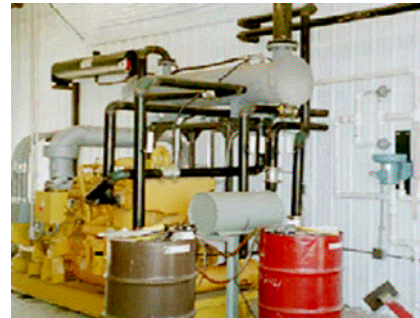
Digester engine with heat recovery system
