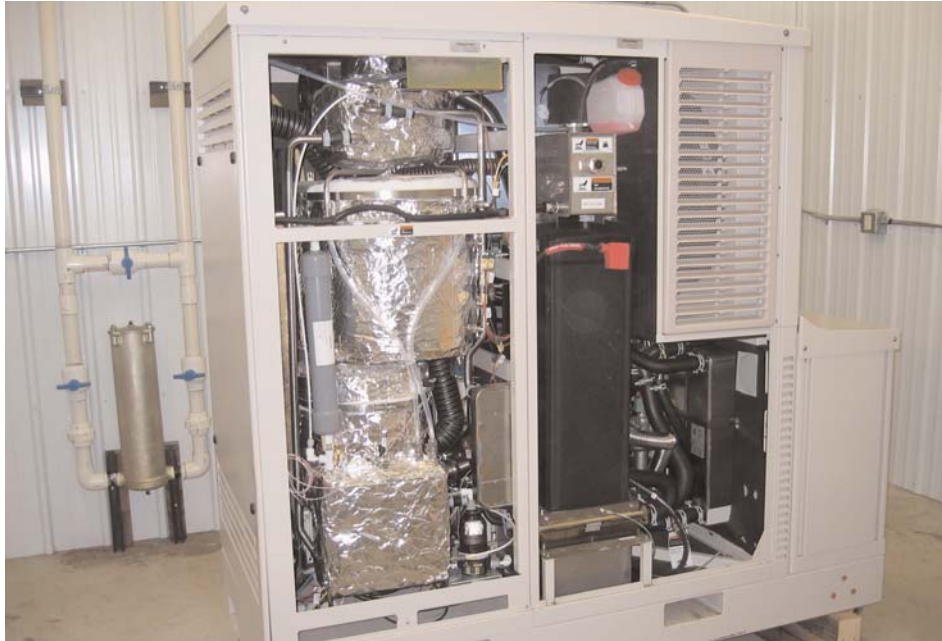
5kW proton exchange membrane (PEM) fuel cell at Haubenschild Dairy Farm
